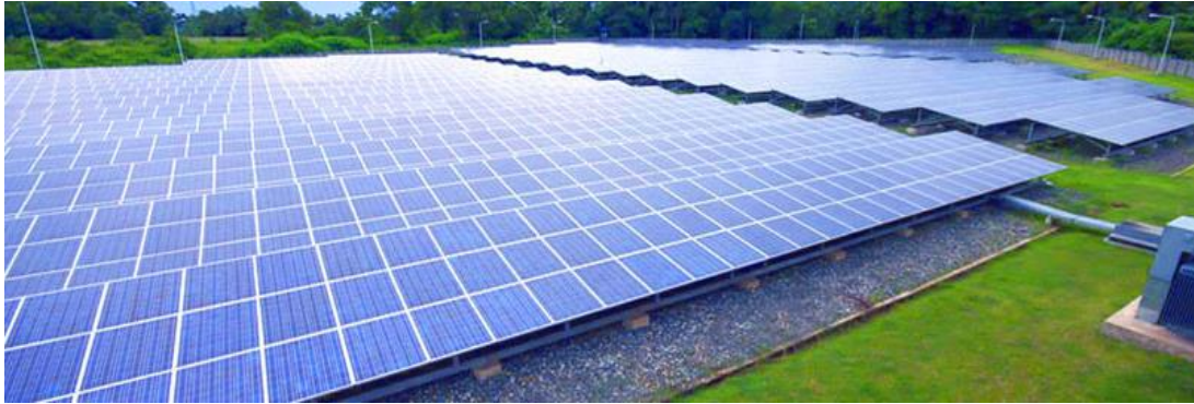
Cagayan de Oro Power and Electric Light Company's solar powered plant (Cepalco, 2014)
